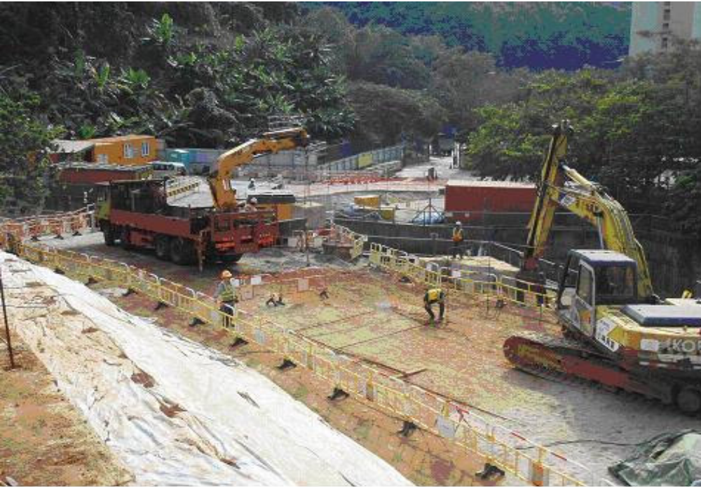
Photographic record for exceedance of Suspended Solid recorded at Sik Sik Yuen Ho Fung College (I-1) on 08-Dec-08
